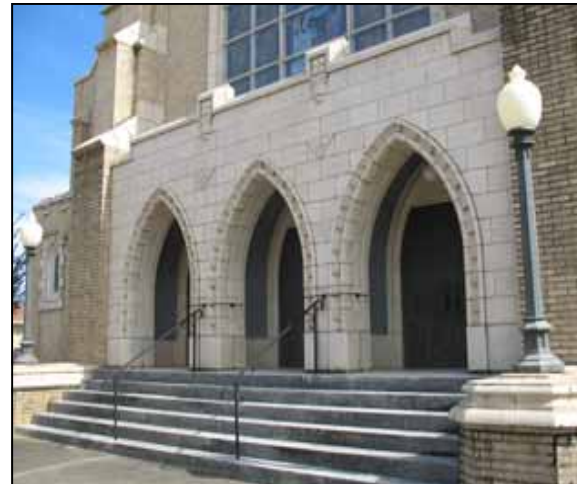
The Centenary United Methodist Church on Delaware Avenue uses a mix of stone blocks for the entrance and cast stone for the detailing on other parts of the church.
