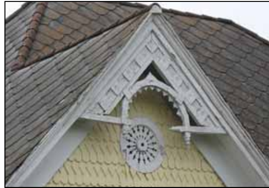
The gable at 530 Third Street features a decorative vergeboard or bargeboard in the upper portion of the gable made up of turned and cut pieces of wood to form a pattern.
