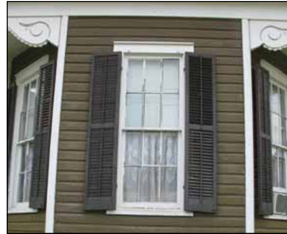
The shutters on this house at 513 Louisiana Avenue are properly mounted on shutter hinges so they close and properly fit the window opening.
