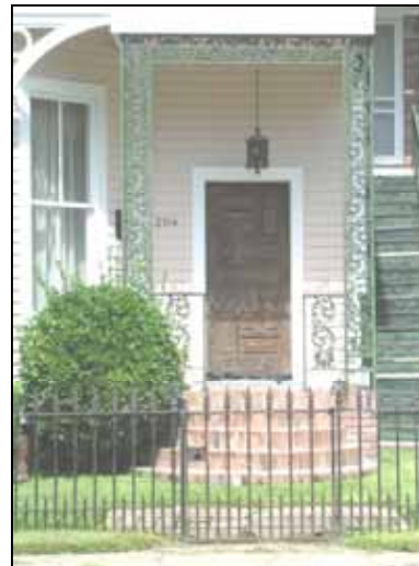
This Queen Anne style house has lost its original corner porch and entrance doorway. The original doorway would have featured a transom and single-leaf door with glazed upper panel. The original porch was enclosed and a new, inappropriate 1970s door with raised panels was installed. Unfortunately, the house also lost its original porch detailing and entrance steps.
