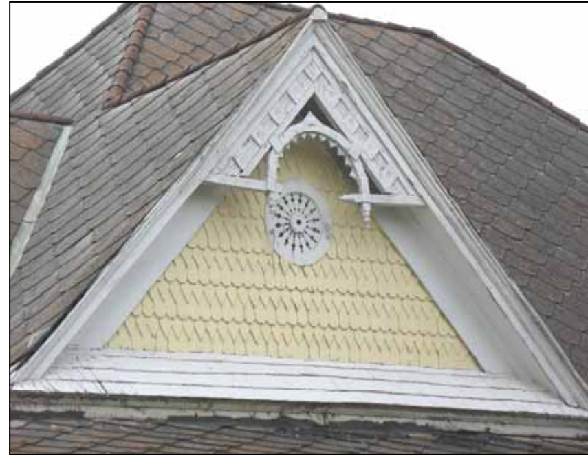
530 Third Street uses a combination of shingle siding patterns in the gable to add visual interest. There are diamond pattern shingles alternating with rounded shingles
