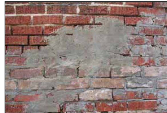
The owner of this brick building tried to stop the mortar erosion and water infiltration by smearing concrete over the deteriorated areas. This makes it very difficult to properly repair the problems in the future and has caused more damage to the brick surface
