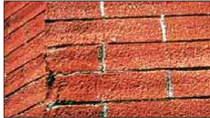
This National Park Service photograph well illustrates the negative effects of sandblasting, which should never be used to clean brick buildings. Sandblasting will not only erode mortar but will also remove the glazed outer surface of brick and hasten deterioration.
