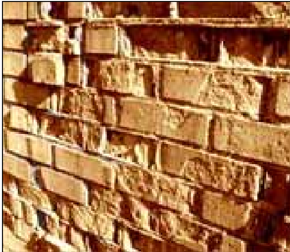
This photograph supplied by Chagrin Falls Preservation in Ohio illustrates the spalling that can occur only five years after using portland cement mortar in repointing.
