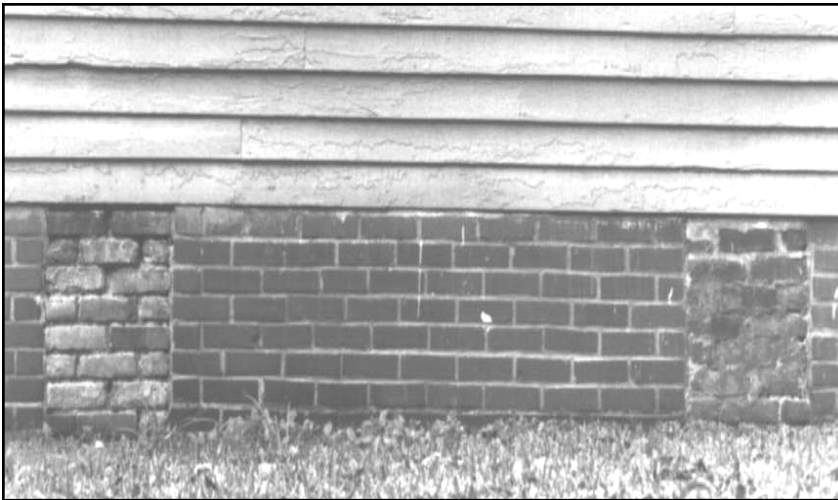
This crawl space enclosure between the original brick piers has altered the historic character of this house and is visually inappropriate. The enclosure also has no vents to provide air circulation beneath the house to prevent the build up of moisture under the house..
