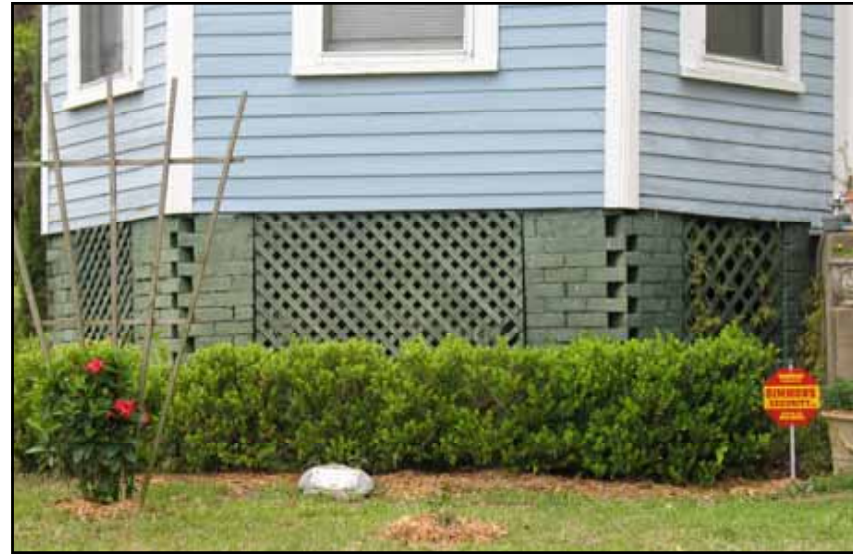
The lattice panels between the brick piers appropriately enclose this crawl space at 430 Third Street.
