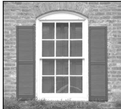
Shutters on this arched window are too short, too narrow, and wrongly hung outside the window frame. Shutters for this window should also form an arch when closed.
