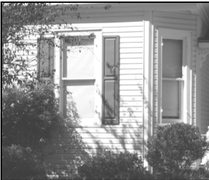
The vinyl shutters flanking this window are too narrow and incorrectly hung outside the window frame. Paneled shutters are also inappropriate for Queen Anne style houses.
