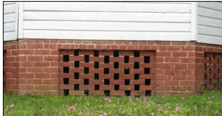
While not as appropriate as wood lattice at least this brick lattice pattern allows the foundation to breathe.
