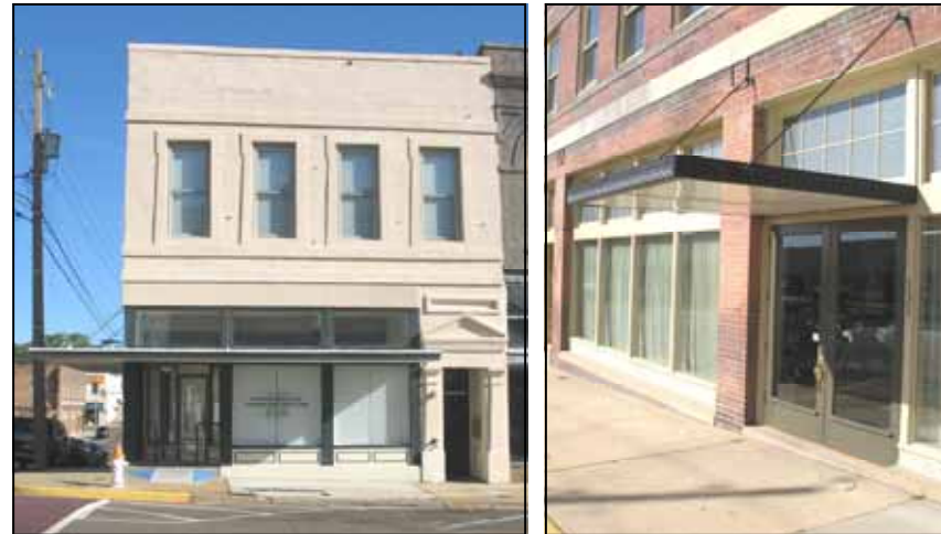
These buildings in downtown McComb show the correct installation and projection for suspended canopies on a commercial building. The projecting flat canopies are anchored by rods which is typical of commercial buildings built in the 1920s to 1940s.
