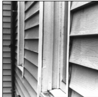
These photographs illustrate how vinyl siding negatively alters the exterior appearance of a historic building. The vinyl siding is nearly flush with the trim around the windows, and J-channels have been installed around the windows to prevent water infiltration behind the siding.
