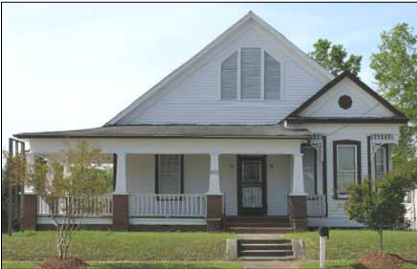
The original columns at 403 Delaware Avenue were most likely turned and later replaced with tapered box columns on masonry piers typical of the later Craftsman style.
