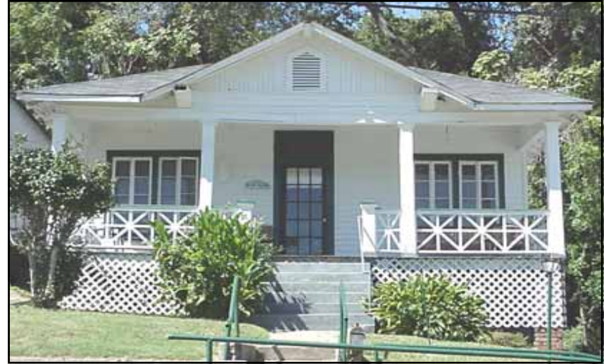
The lattice used to enclose the crawl space beneath this historic house in Natchez is inappropriately installed, because it overlaps and obscures the brick supporting piers.
